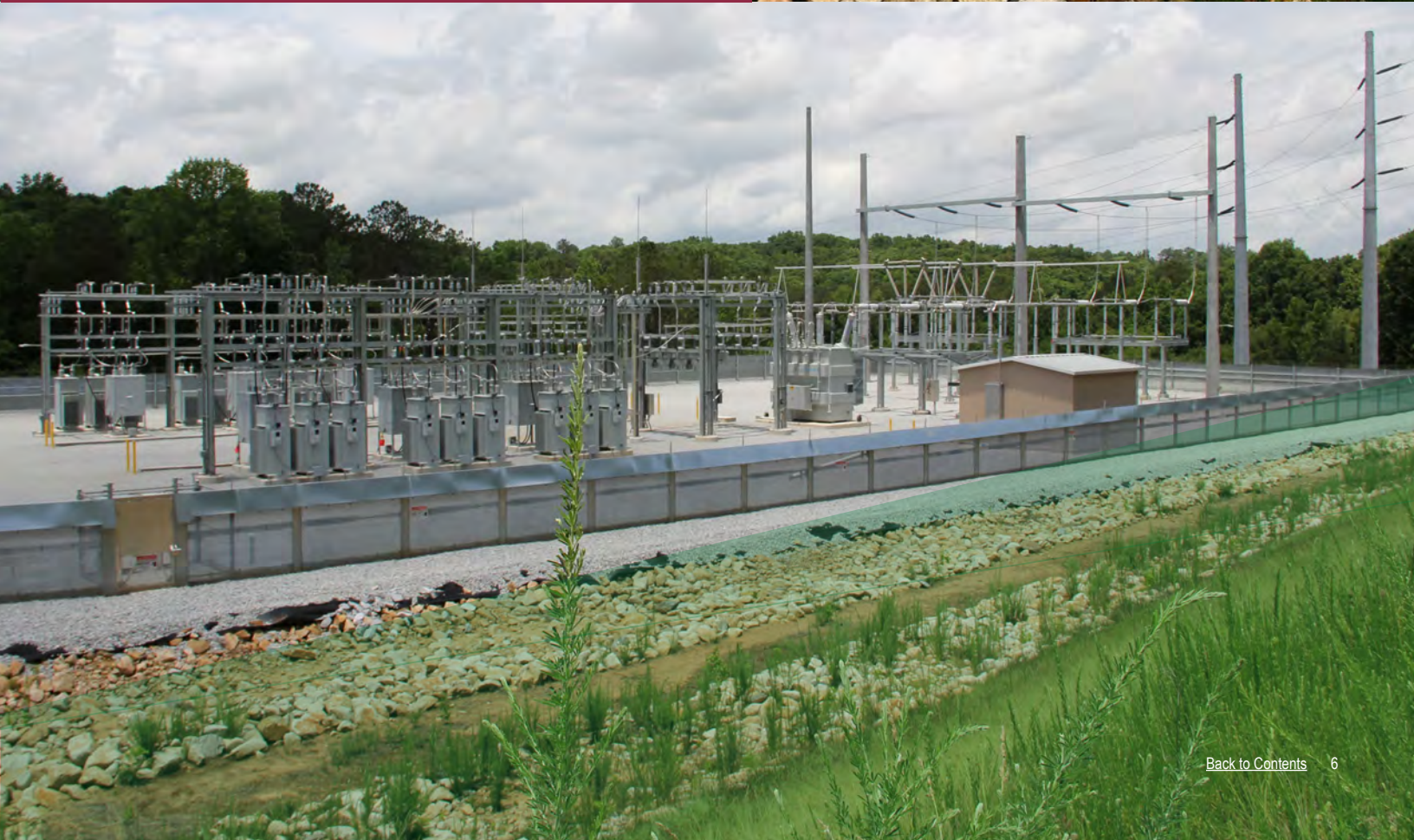
For the Wolf Creek Substation, a plateau was constructed to provide a stable foundation with a front wall soaring to a height of more than 50 feet.
